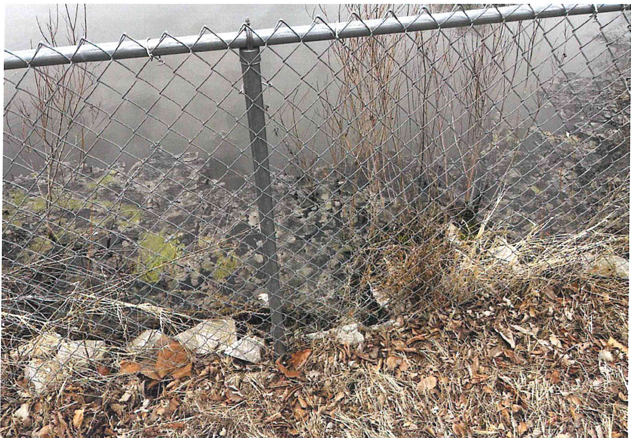
Eroded bank on east side of detention pond
