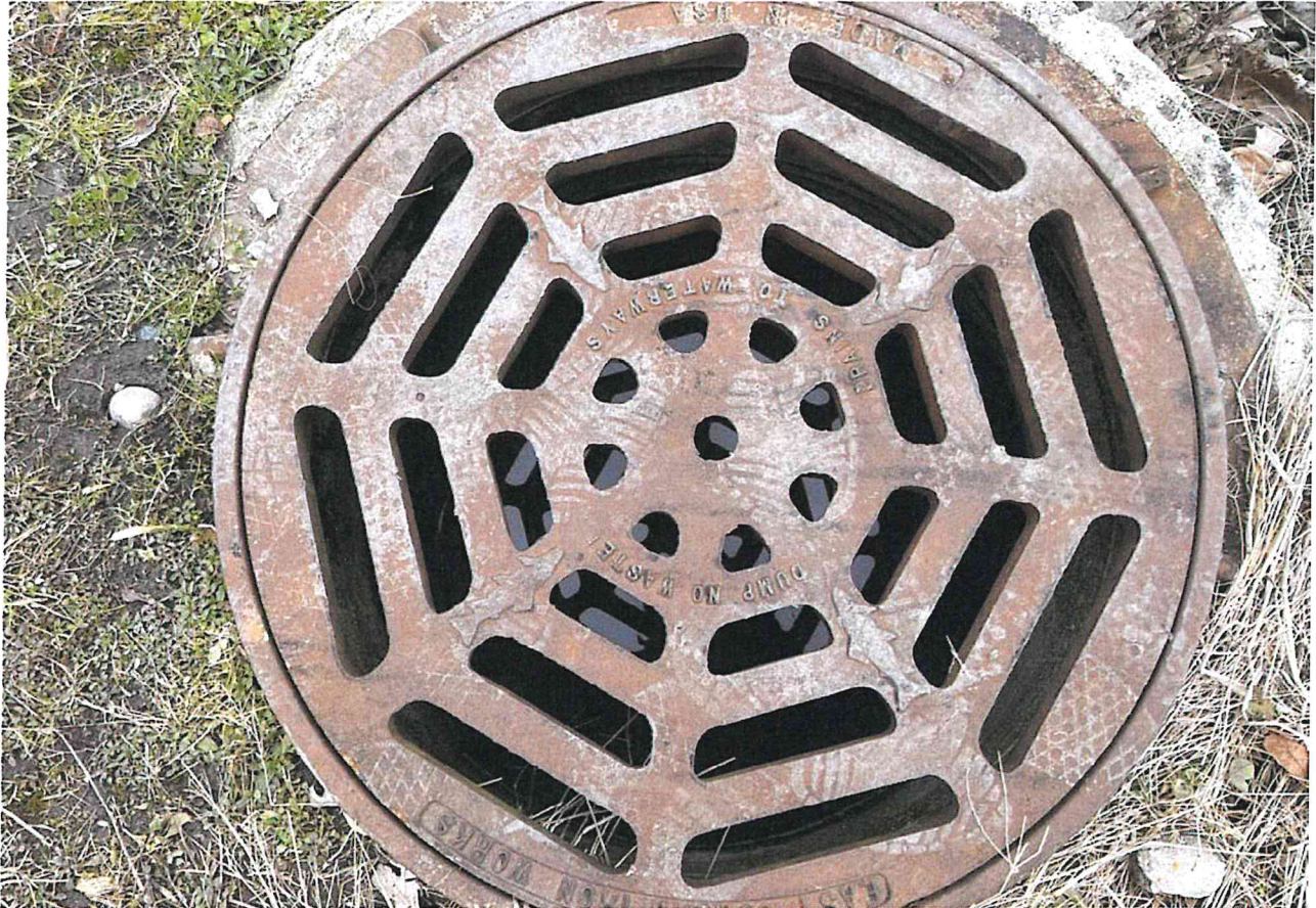
Standing water and submerged pipe in catch basin
