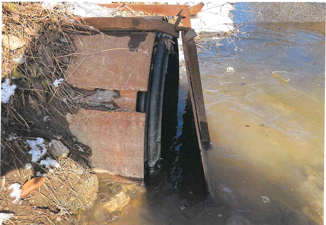
Flap gate unable to close or open due to sediment and damage
