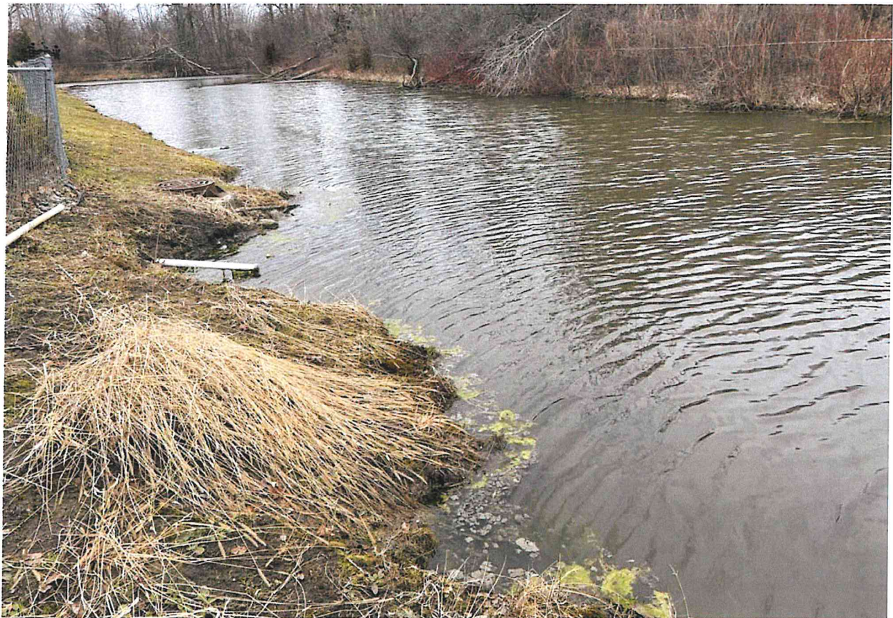
Erosion on south bank of detention pond
