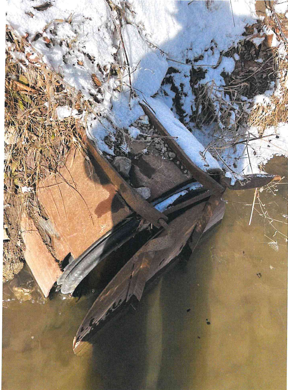
Damaged flap gate
